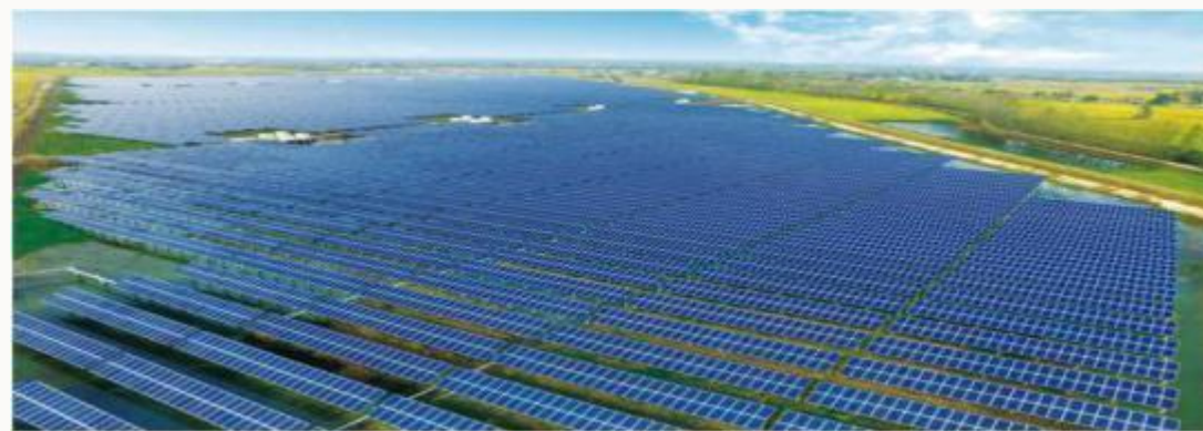
40MW fishing-solar complementary PV plant in Shitang, Hefei
