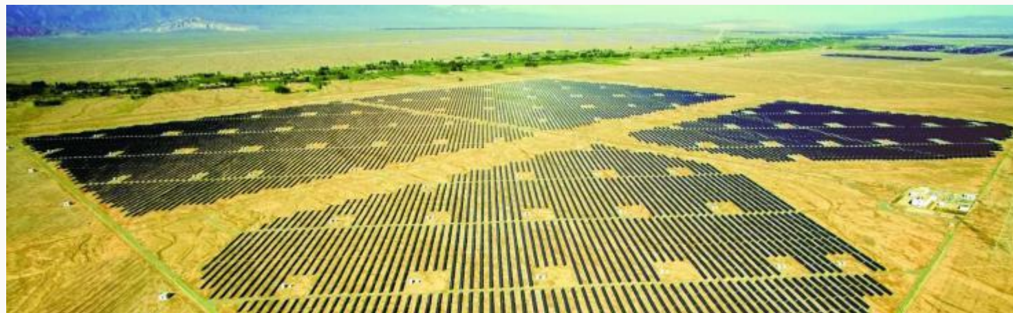
100MW utility PV plant in Jiuquan, Gansu
